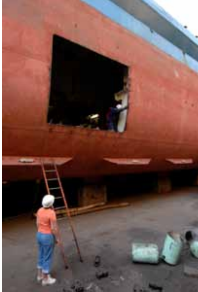
Large holes were cut in the side of the Africa Mercy in order to install the new generators
